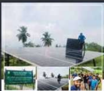
Agunakolapelessa Solar Powers System
